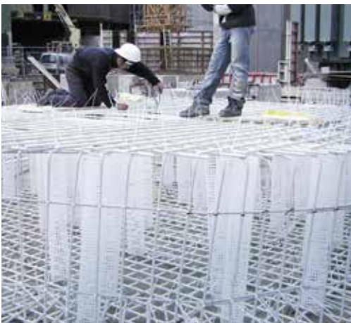
Foundation reinforcement in the switchgear house at Peiner Träger GmbH, Peine, Germany
