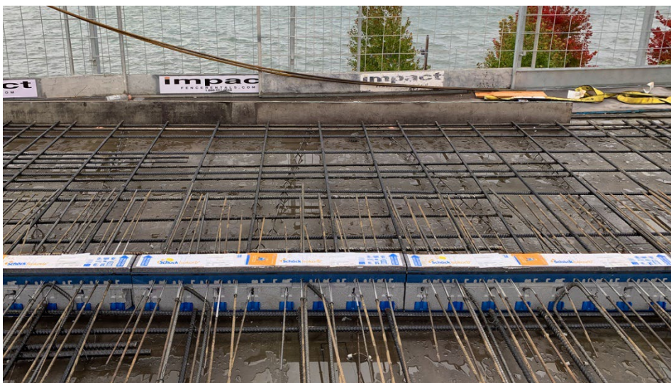
Structural thermal breaks are secured to the rebar on the balconies and interior slabs.
