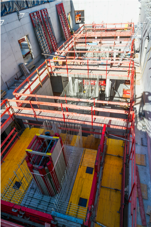
A total of four high-precision measuring rooms will be erected at the ZAQuant. Photo: Schöck Bauteile GmbH, reprint free of charge.
