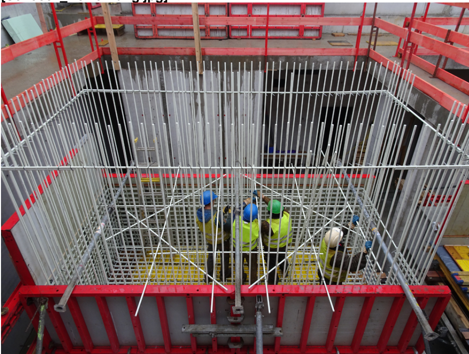
The high-precision measuring rooms will be reinforced with Combar. Photo: hammeskrause architekten bda, reprint free of charge.
