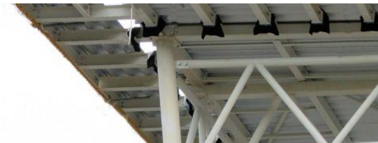
The KST modules in position
