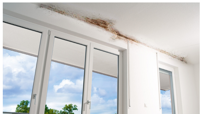
Condensation forming on the underside of an uninsulated balcony penetration can lead to mold growth, respiratory problems and litigation in modern, air-tight buildings having interior humidity levels exceeding 35%.
